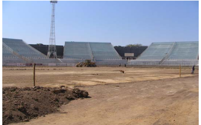
There was considerable excavation work to put the perfect foundations in place.
