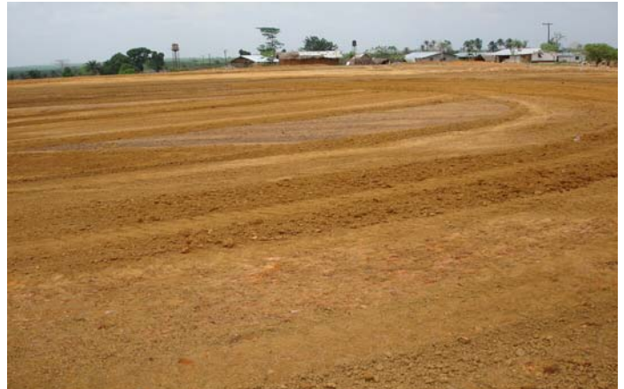
The ground being prepared for the installation of an all-weather artificial football turf pitch.
